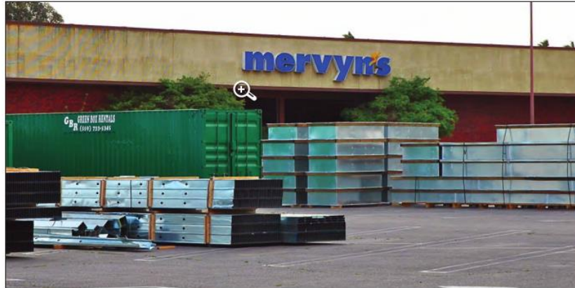
CHUCK HARVEY | Walmart expects to complete the refurbishing of a former Mervyn's location in Central Fresno by the summer. The 107,000 square-foot building has been empty for five years.
